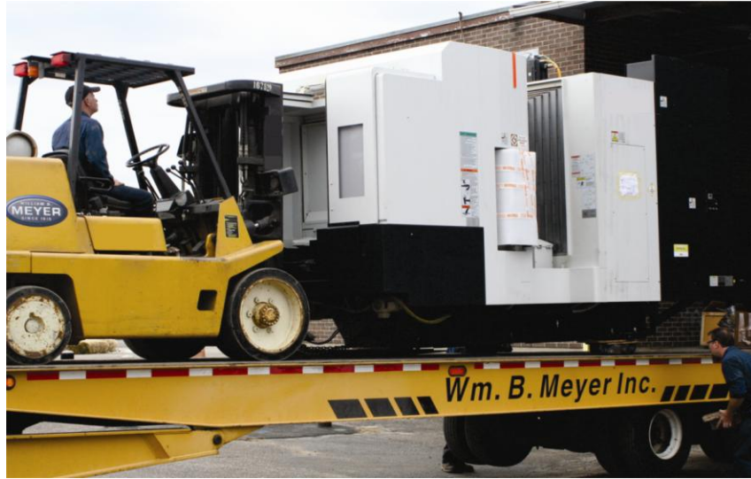
Figure 1: Specialized equipment and skilled personnel provided by MEYER Rigging ensure successful machine installation at Tier ONE.
